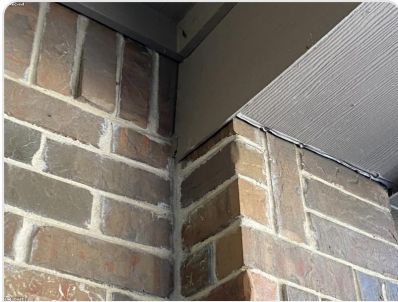
West side — soil slopes back toward the foundation wall.
