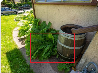
NE downspout ends at the foundation — extend 4–6 ft.
