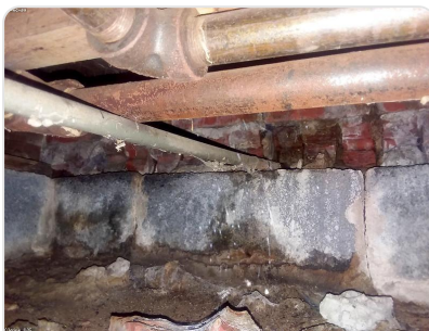
Vapor barrier displaced at seams — bare soil exposed.
