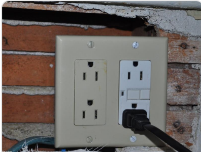
Kitchen counter receptacle — no GFCI protection present.
